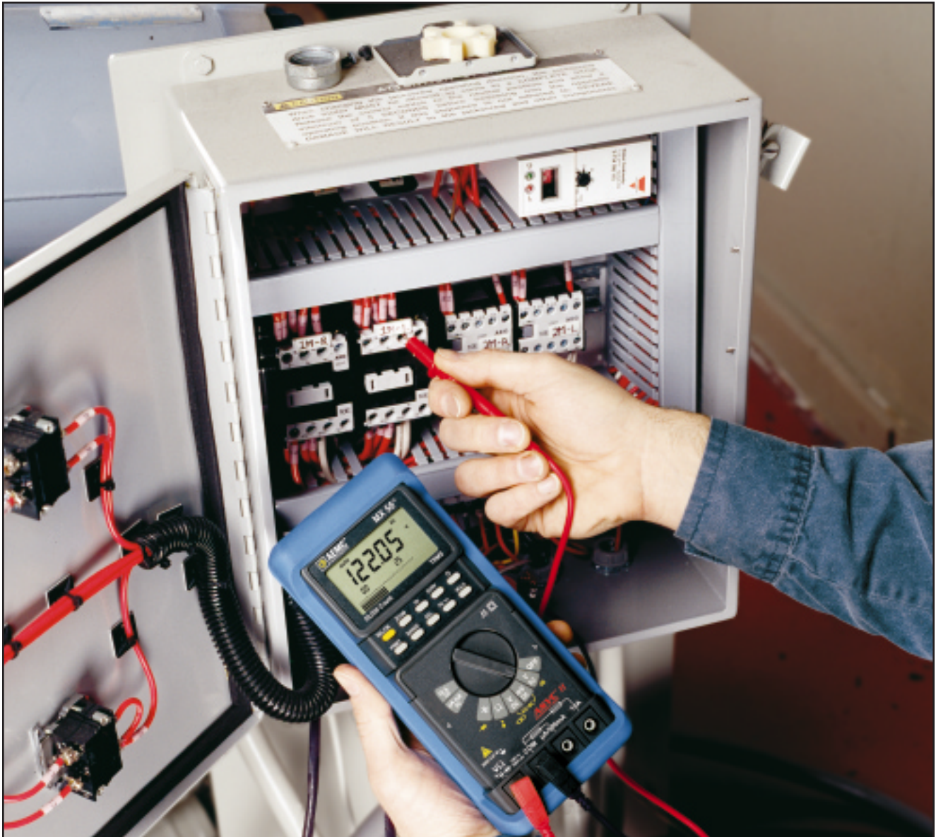
Model MX56 III measuring DC voltages in a signal control panel.
