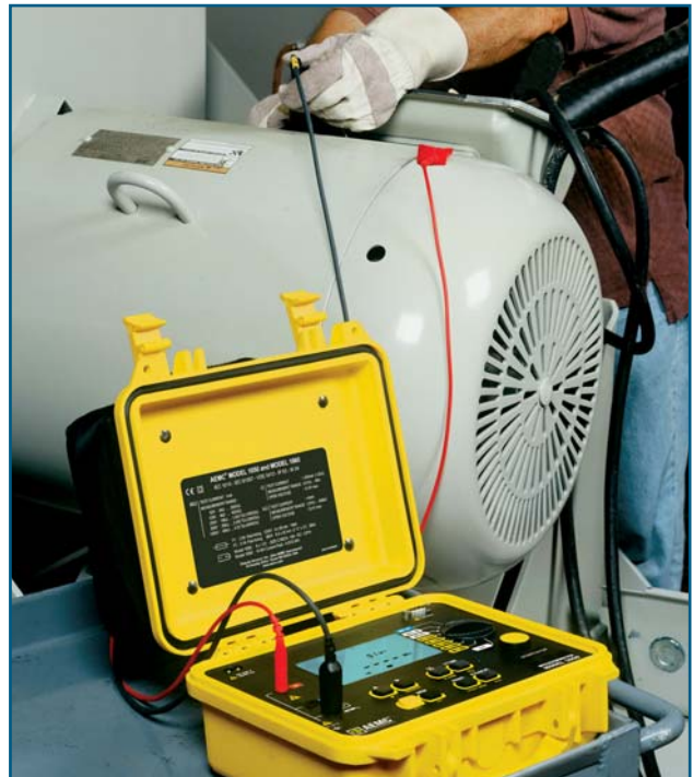
Model 1060 checking insulation resistance between windings on a three-phase motor.
